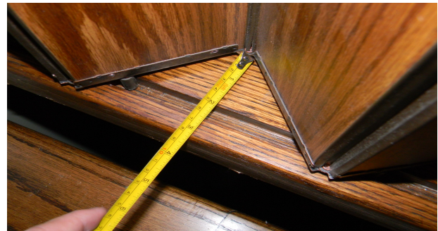
Figure 4. Space of an elevator can entrap children
